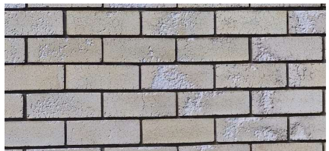
the white staining in the walls
